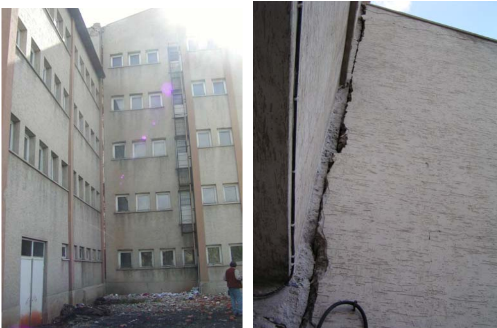
Figure 6. Close-up View of Building Joint in Bingöl
